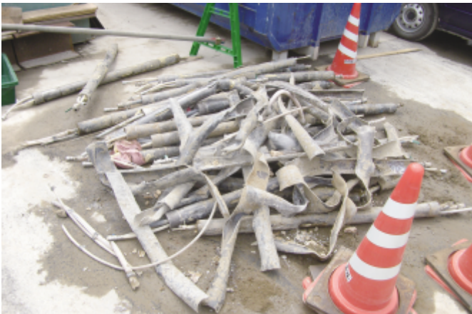
Status of separation and collection of steel piping used in the excavation of tunnels
